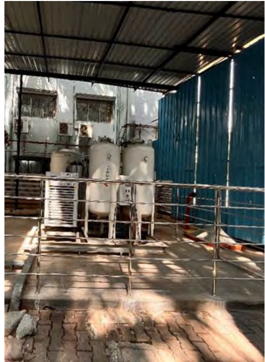
Figure 210: Oxygen Plant Setup Under the Support from Infosys Foundation
